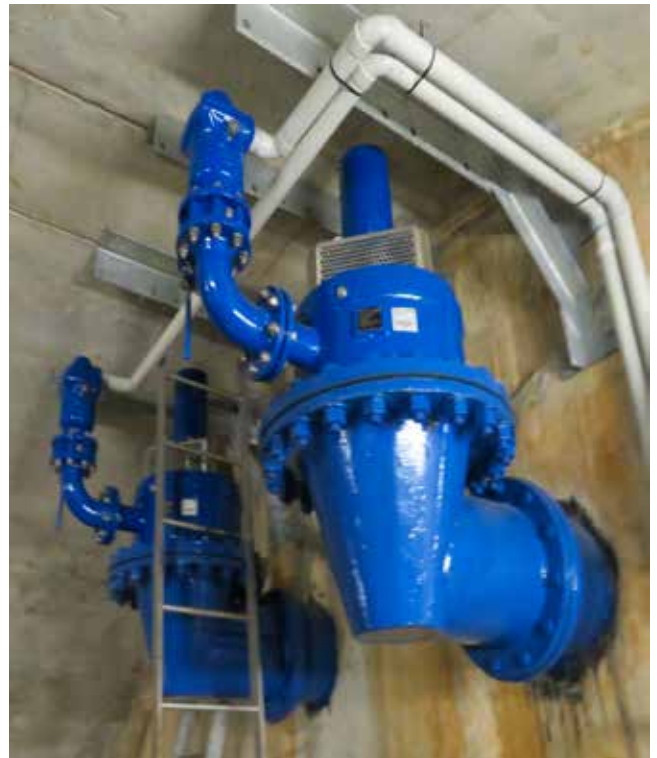
DN 600 Anti- Vacuum Air Valves Installed at a dam in Victoria
