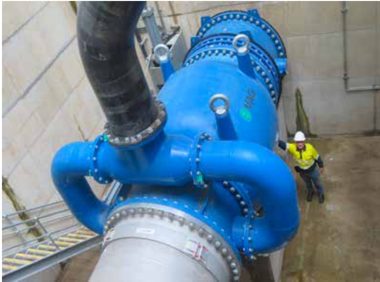
VAG/Metaval successfully supplied and Installed a DN 1800- Plunger valve with aeration and VAG guard valve plus VAGS dismantling joint ( all DN 1800). This is the largest plunger valve to be installed and successfully operating in Australia .
