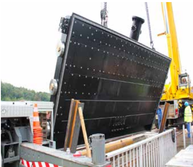
ROLLER GATE 10mts x 5 mts
